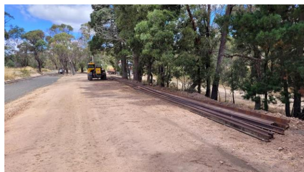
Rail for turn out at Hazelgrove, NSW.
