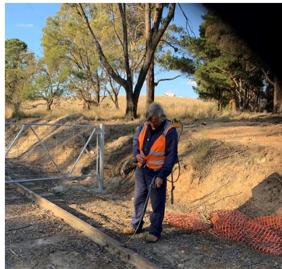
A new addition to the maintenance program. Mark ensuring the rail joints are well lubricated and the fish pate bolts are not overtight.
